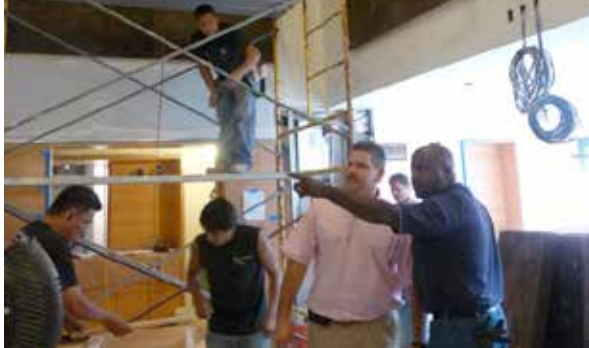
Two program mentee firms, First Choice Mechanical and Corinthian Construction Company, working together on a project
