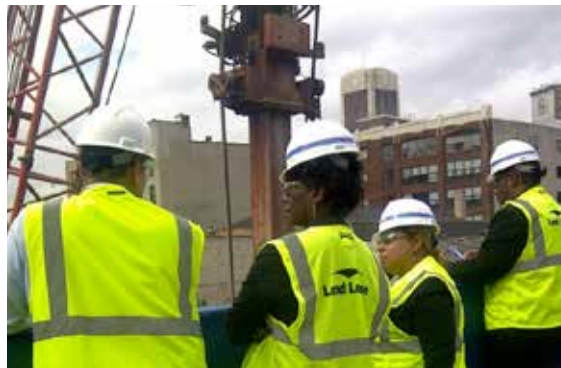
Members of the MWL Construction Advisory Council receive a tour of the Manhattanville Construction site
