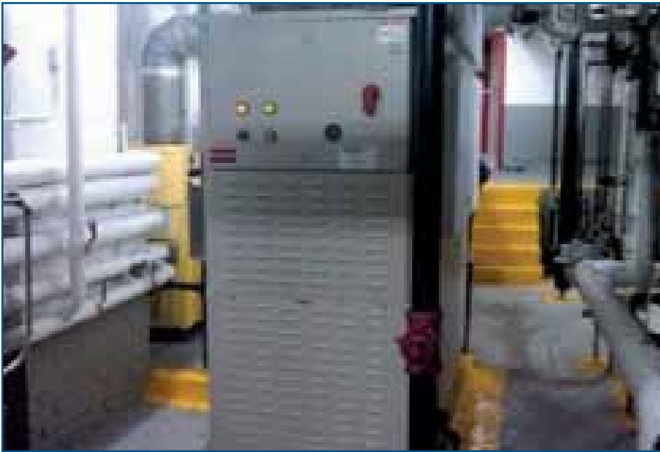
Microturbines, like the one above, will help generate electricity and heat water in Columbia University's residential housing.
